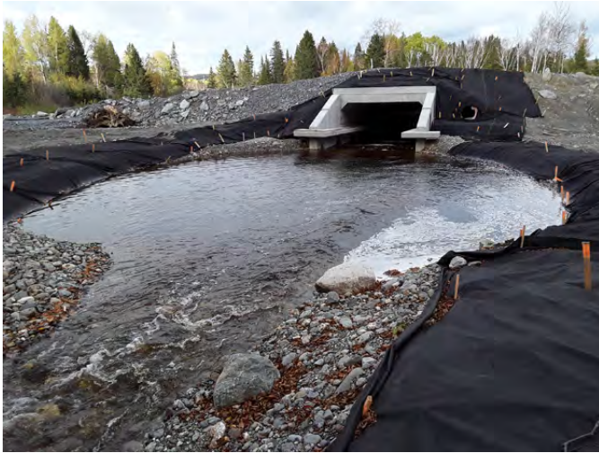
Figure 3. Shelved culvert for small to medium size mammals on Highway 85 (Credit: Ministère des Transports du Québec).
