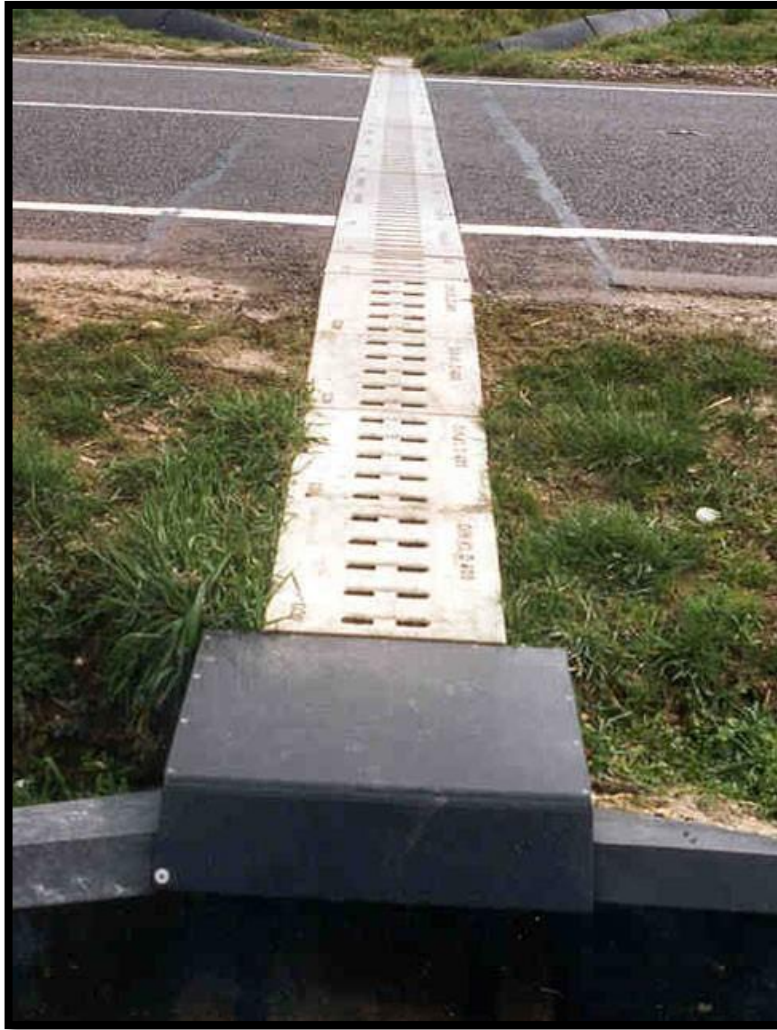
Figure 34. ACO polymer concrete tunnel that maintains more natural ambient light, temperature and moisture conditions through a grate system that lies flush with the road surface. (© ACO Wildlife)
