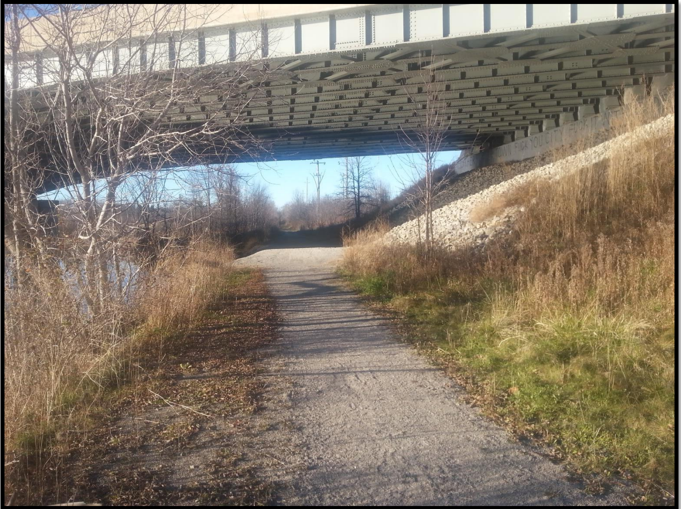
Figure 21. Gananoque River Bridge showing the Gananoque Waterfront Trail on the river's east side. (© Clayton Shearer)
