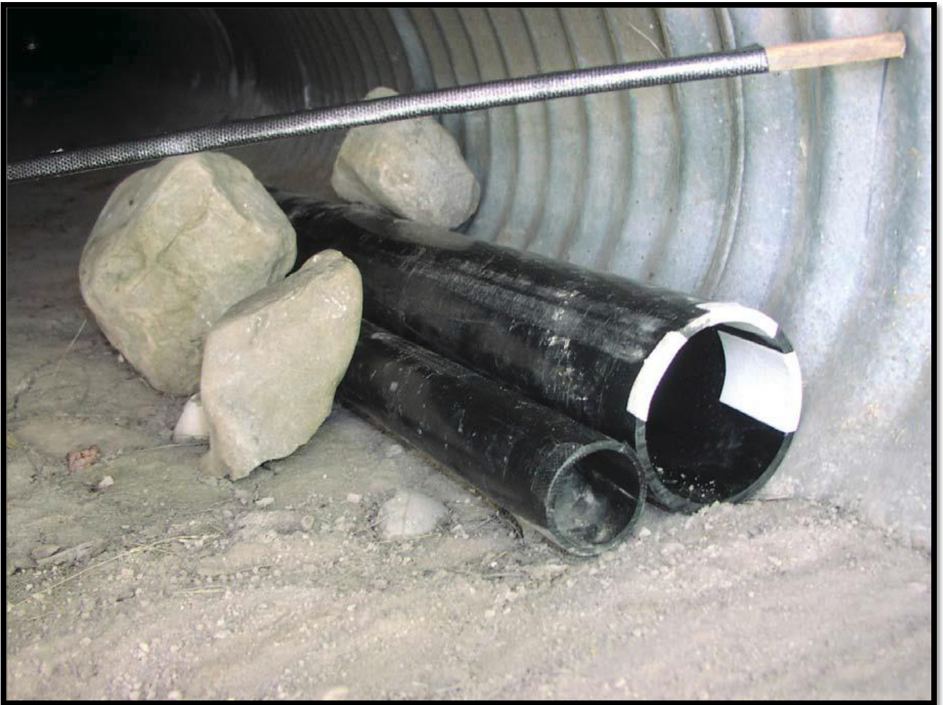
Figure 35. PVC pipes placed in a corrugated steel pipe culvert to provide passage options for herpetofauna and other small wildlife. (© Tony Clevenger)
